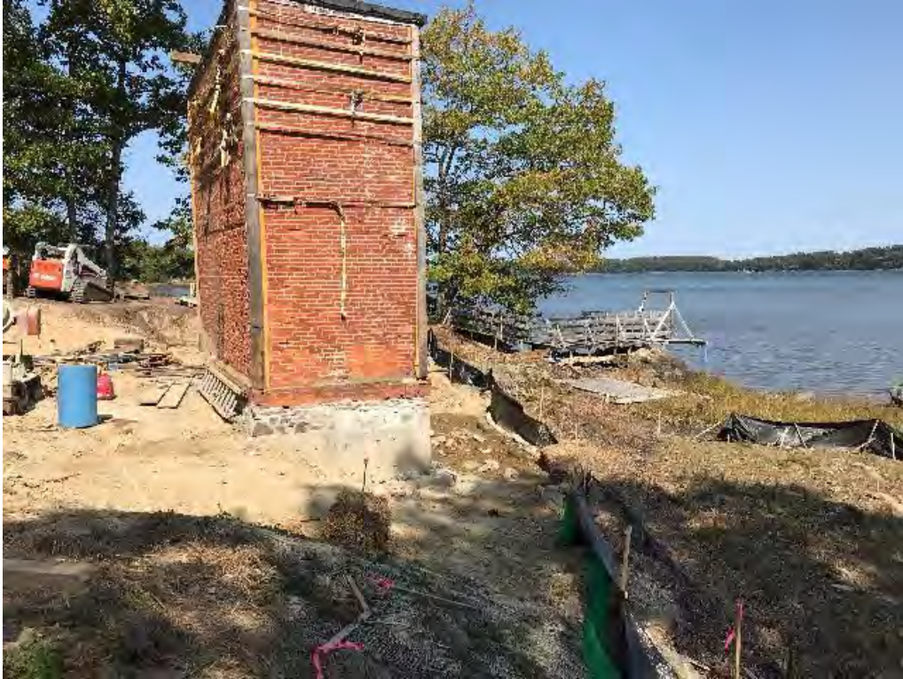
Fig 1: Cable house at Eversource property/west side of the bay. Viewing north. (09-23-20)
