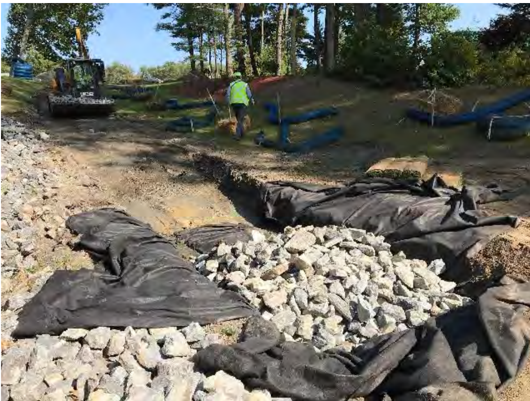
Fig 6: Beginning installation of the subsurface drainage system at Gundalow Landing/east of the bay. Viewing east. (09-23-20)
