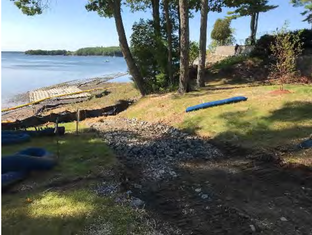
Fig 3: Stone removed from slope below the manhole at Gundalow Landing/east side of the bay. Viewing west. (09-21-20)
