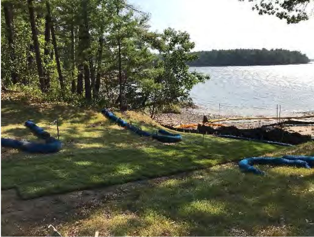
Fig 5: Installing sod on the slope below the manhole at Gundalow Landing/east side of the bay. Viewing south. (09-23-20)
